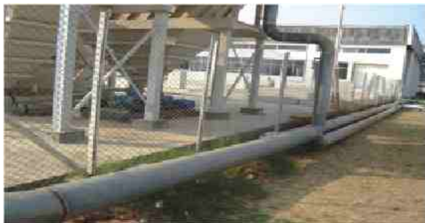
Natural Gas Supply Pipelines
